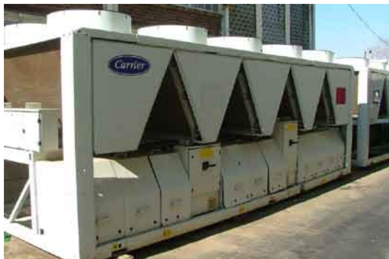
Air Cooled Chiller 652kw
